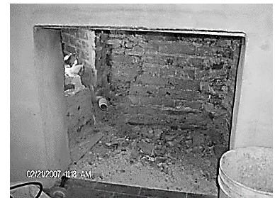
Badly Deteriorated Firebox
