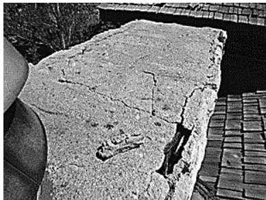
Damaged Chimney Cap
